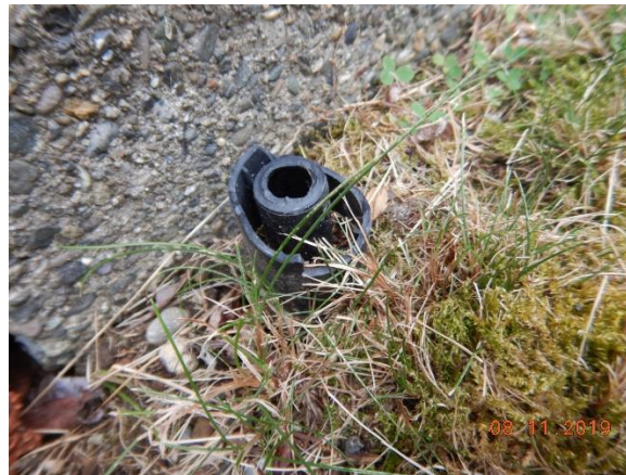
Damaged irrigation head
