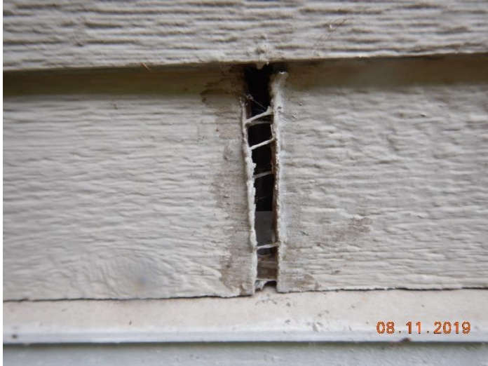
Gaps at the end joints should be caulked
