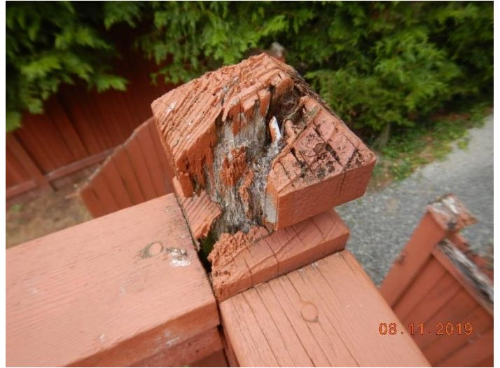
Rotting barricade post (typical)
