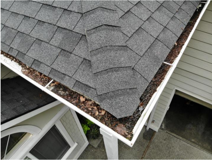
Debris in the gutter above the entryway
