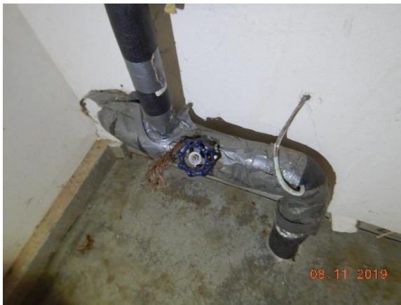
Domestic Water Shut off
