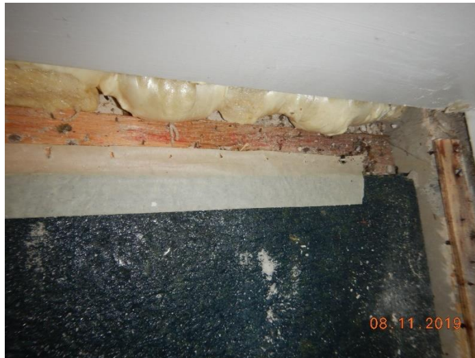
Settlement of 2" +/-; expansion foam has been added. The carpeting was unsecured at the outer corner of the room
