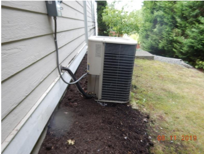
The compressor is not level
