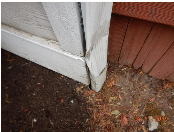
A downspout at the rear of the home is crushed, however appears to service its intended purpose
