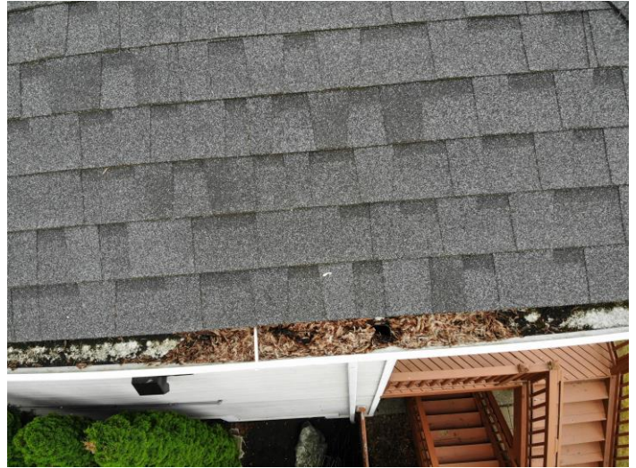
Debris at an upper rear gutter
