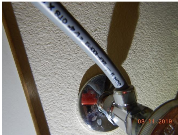
Polybutylene pipe @ sinks
