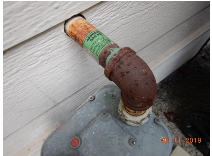
Rusting gas pipes
