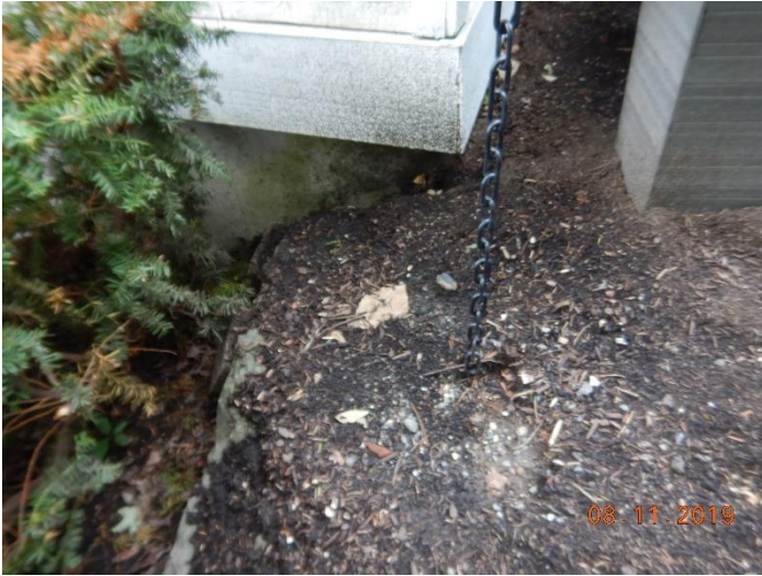
Downspout chain. No splash-block or drain is provided (WDO conducive condition)
