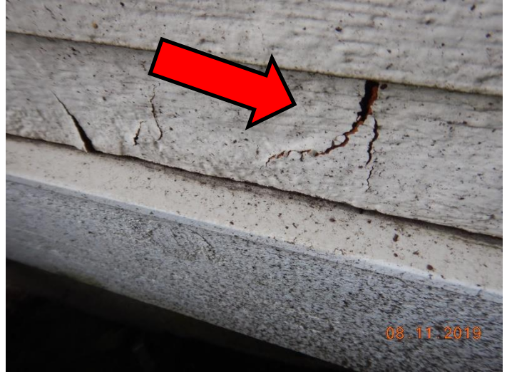
Failed siding at the Living room area
